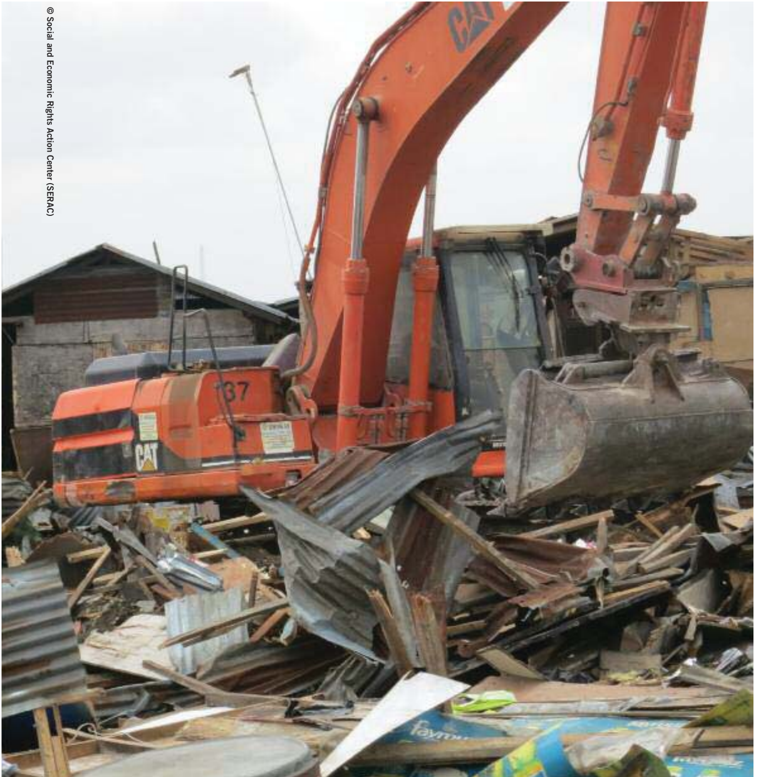
A bulldozer demolishing homes in Badia East. On 23 February 2013 at least 266 structures were demolished by the Lagos state government. There was no genuine consultation and reasonable notice before the demolition.
