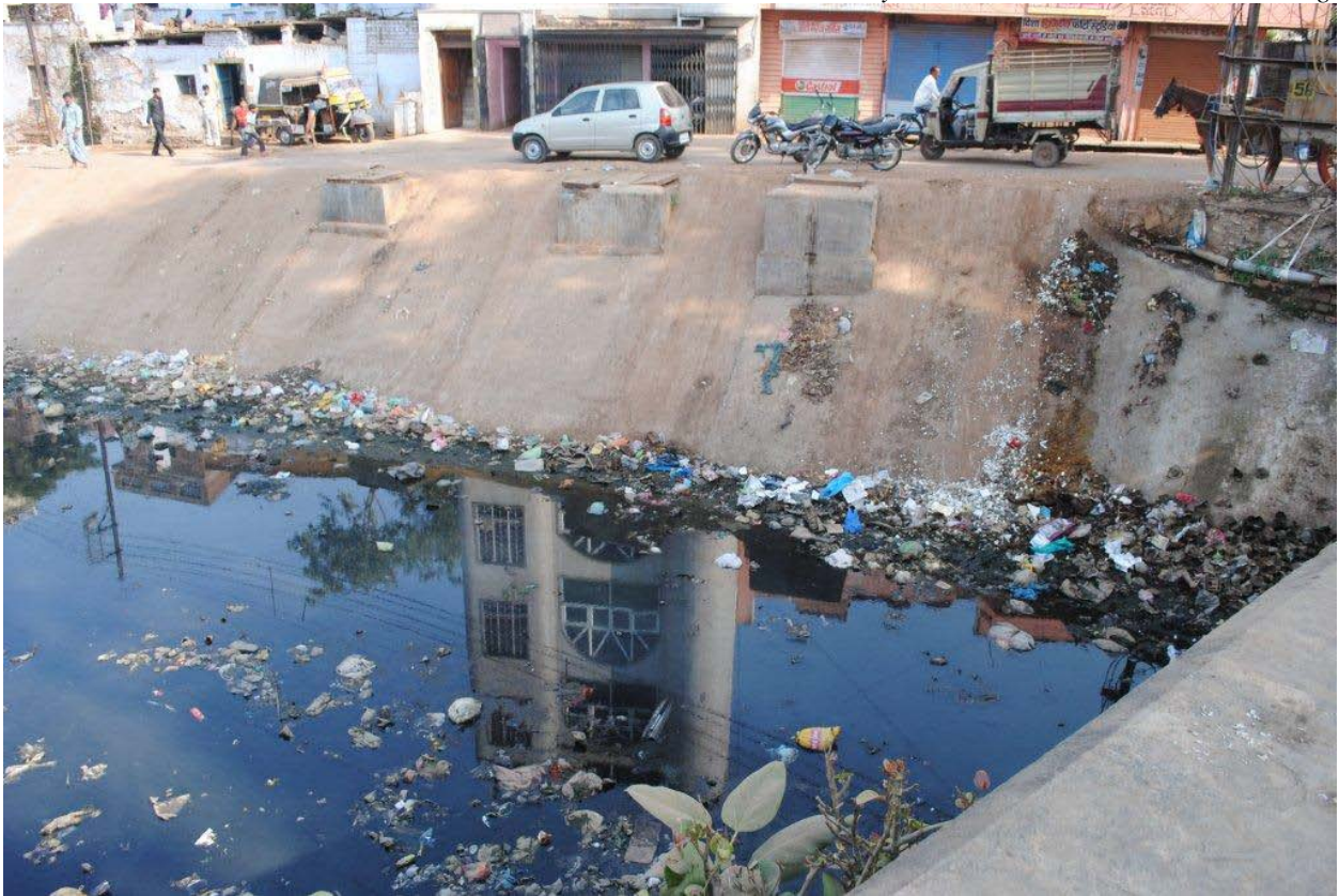
Photo 5. October 2010: Accumulation of debris due to lack of cleaning
