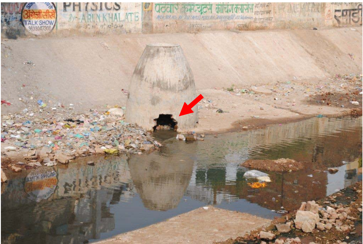
Photo 6. October 2010: Broken manhole releases sewage into the river.
