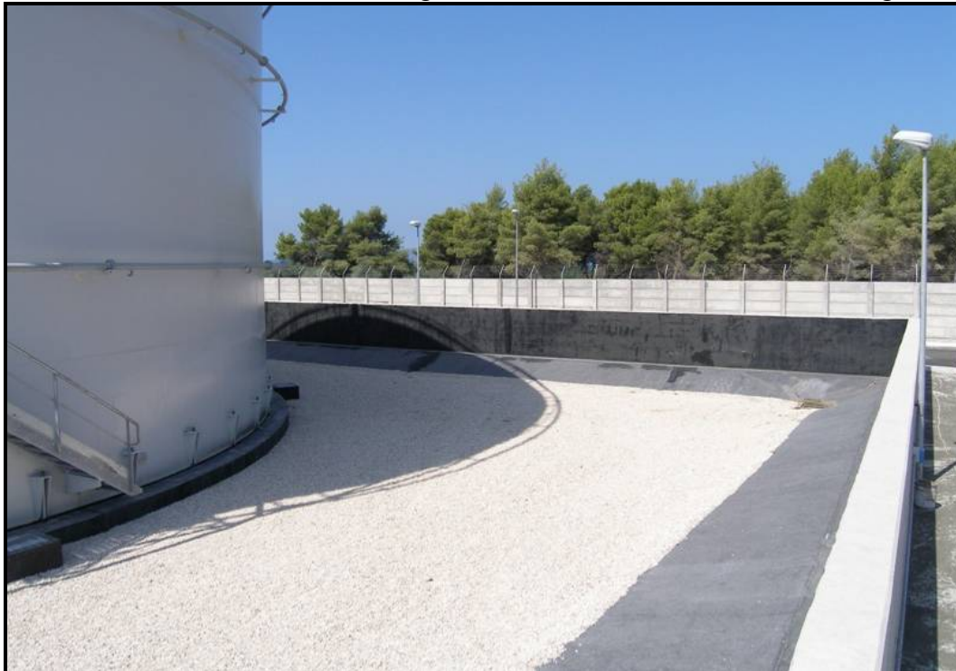
Photo 7. Spill containment around oil storage tank
