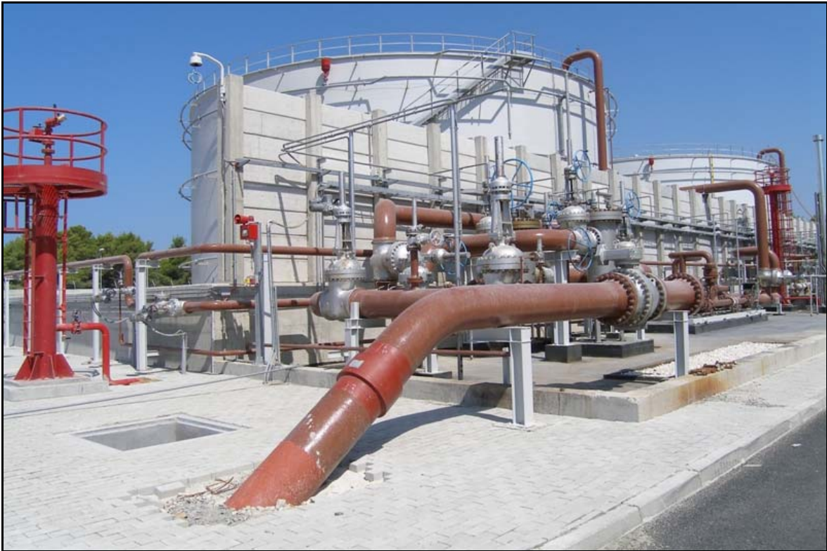
Photo 8. Oil pipeline hook-up at plant (valves and spill containment at base)
