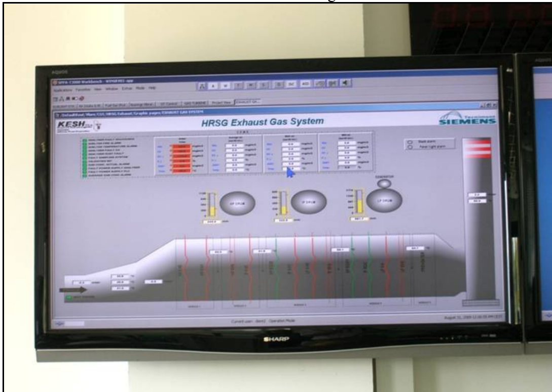
Photo 5. Readout of air monitoring station in operator room (indicative since plant not yet operational)
