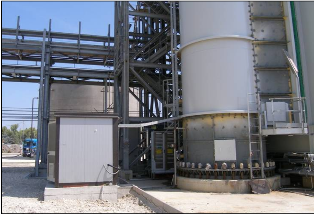
Photo 4. Continuous air monitoring station near stack
