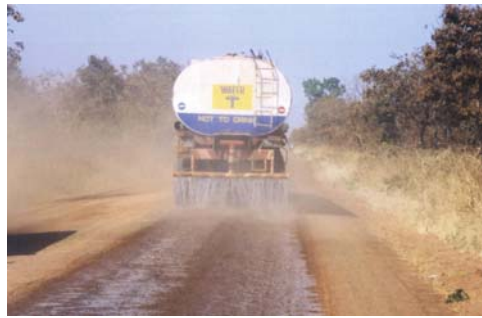
Picture 6: Mitigating dust impacts generated by newly constructed roads for the Project
