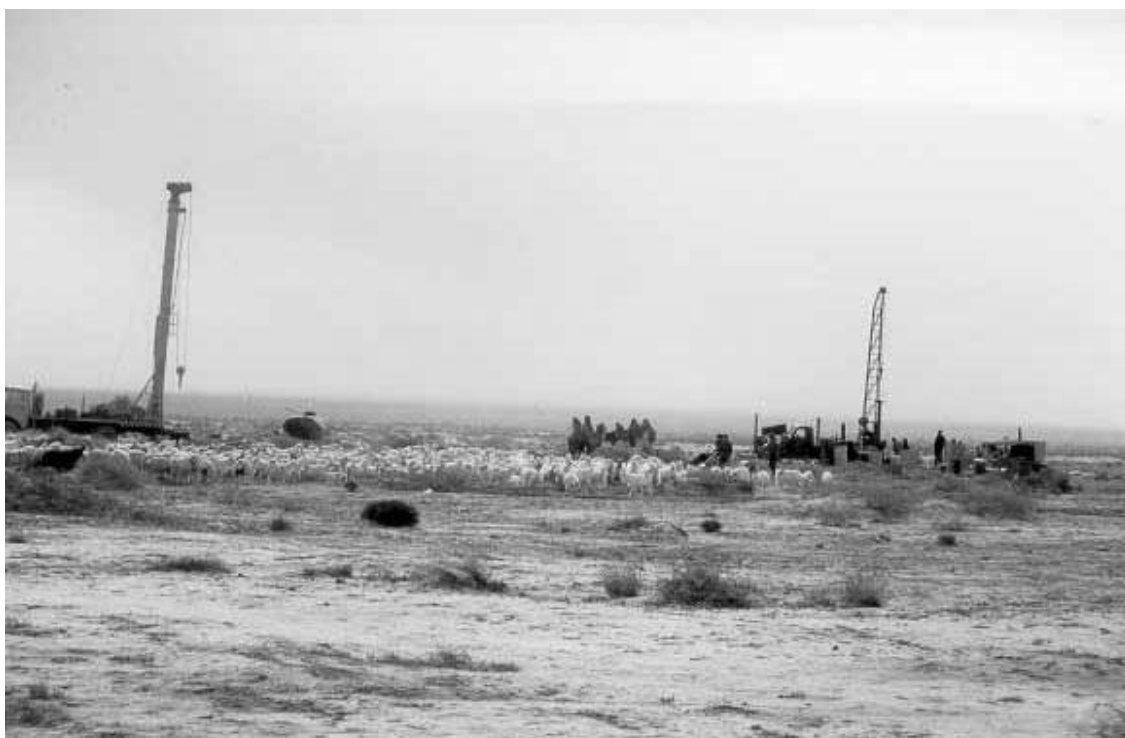
Figure 15. Drilling rig observed on October 15, 1999, at the site of the proposed Xiangride-Balong Irrigation Sub-district.
