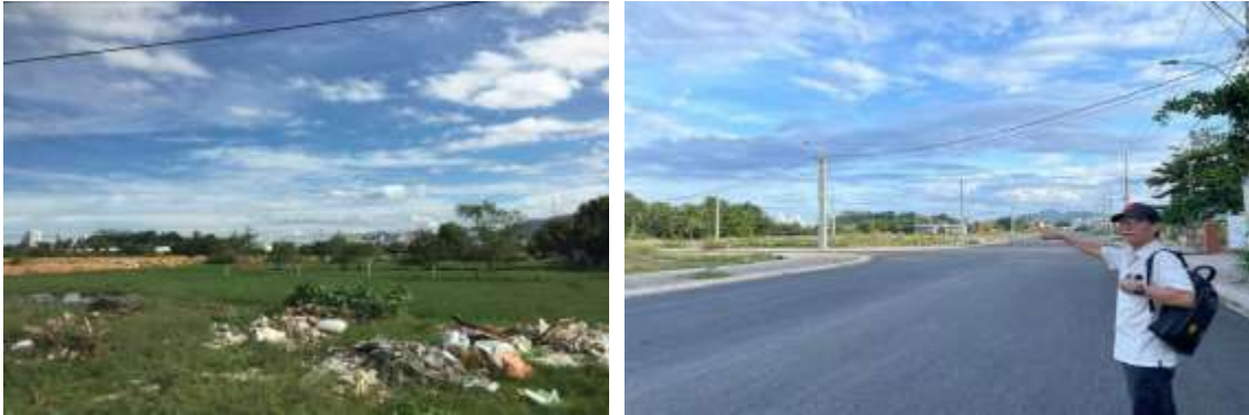
Photos 5 and 6. The Ngoc Hiep site (8.5 ha) before (left) and after (right) infrastructure development.
