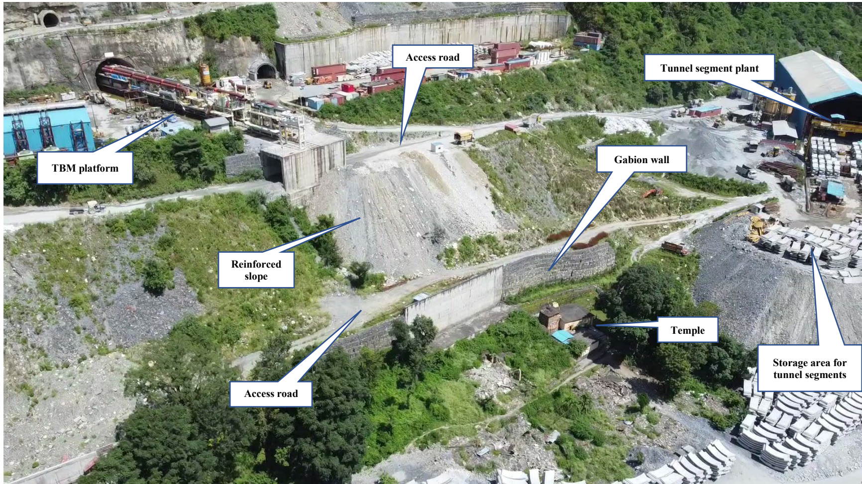
Photo 1: Aerial photo of the temple complex and the surrounding project works (August 26, 2022). No muck is being dumped behind the wall to the north of the temple complex (i.e., behind the gabion wall).
