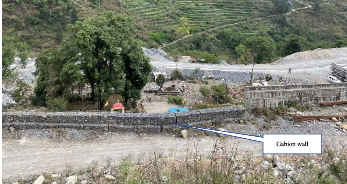
Photo 4. View of the back of the gabion wall (red roof of temple complex visible) showing that no muck is being dumped behind it
