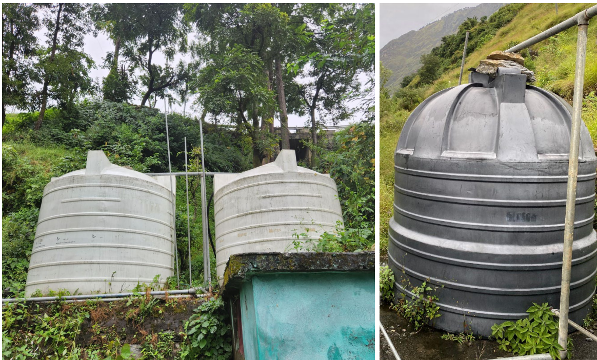
Picture 3: Water tanks in Eldana and Daswana.
