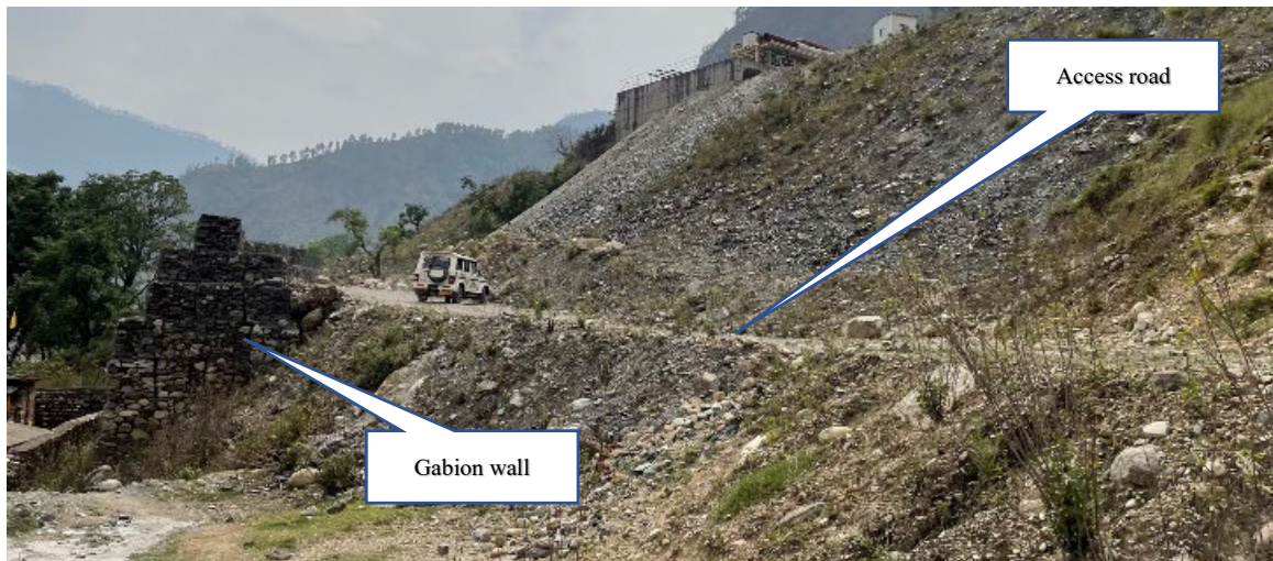
Photo 3. Cross-section view of gabion wall with access road to the right and temple complex (not visible) to the left. If the gabion wall was used to protect against stored muck, this access road would not be usable by vehicles.
