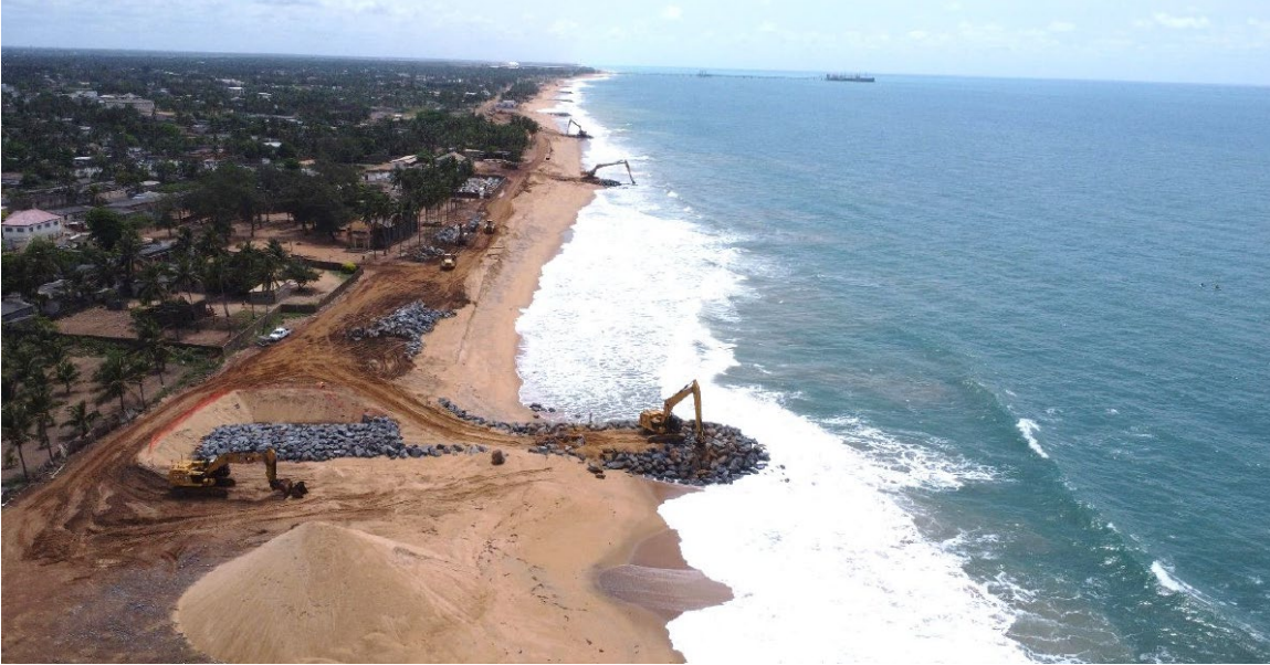
Photo 3. Example of groynes under construction to address erosion (March 2023). When finished (expected June 2023), the area in between the groynes will be filled with sand (Agbodrafo, Togo).
