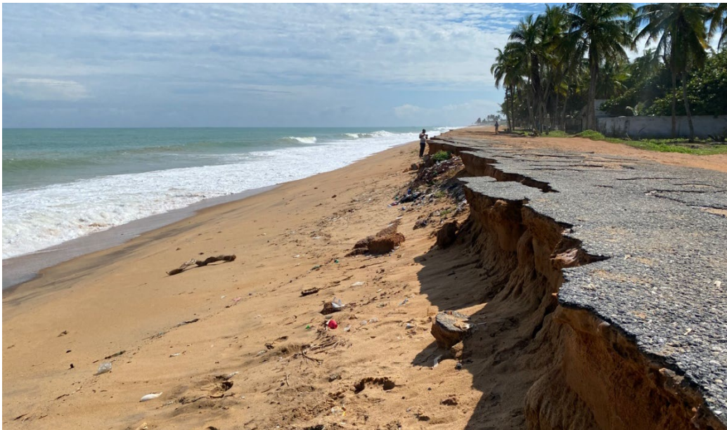
Photo 2. Remnants of the Lomé-Aného Road lost to coastal erosion (June 2022)
