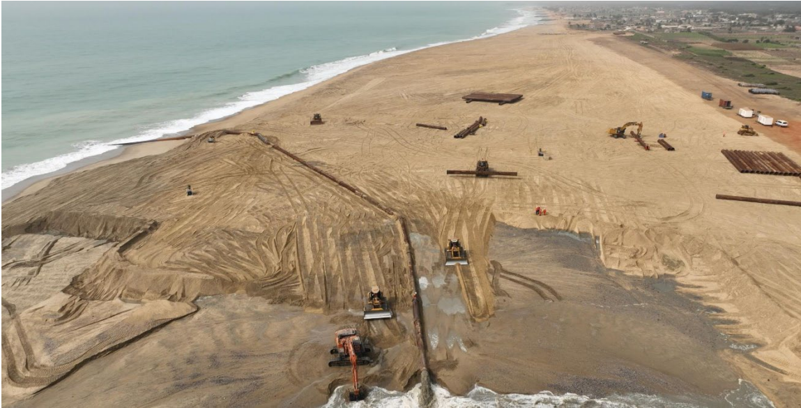
Photo 4. Beach restoration by pumping sand on the shore in Benin, which is part of the Togo-Benin coastal protection solution (March 2023)
