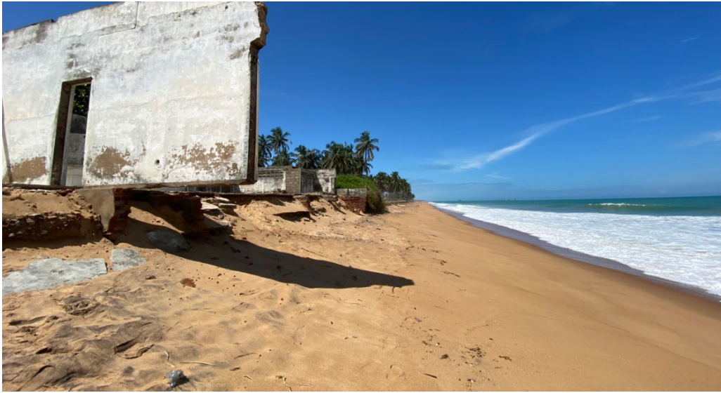
Photo 1. Receding shoreline evidencing coastal erosion in Togo (June 2022)
