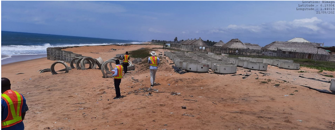
Picture 6. Emergency coastal works to protect livelihood assets (a small resort) is almost completed. Surplus construction material will be removed (September 21, 2021)
