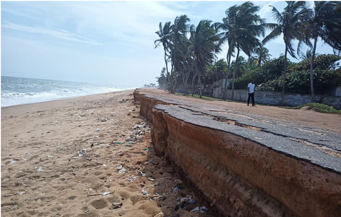
Picture 2. Remnants of the eroded Lomé-Aného road
