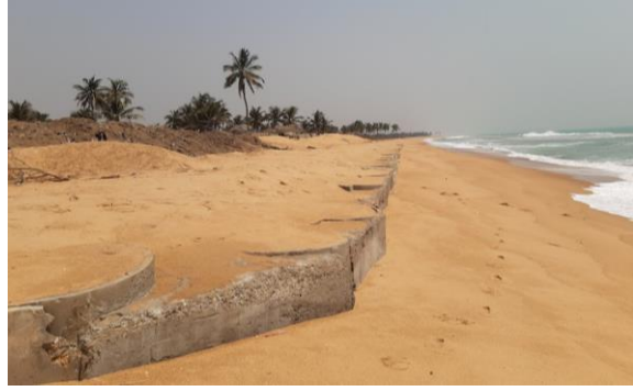
Adissem: view of the extension of the works to the East from the Eastern corridor
