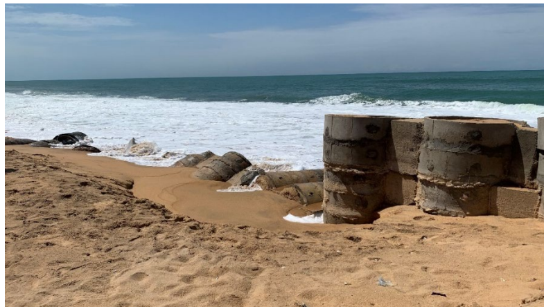
Picture 1: Collapsed concrete pipe wall in Tango
