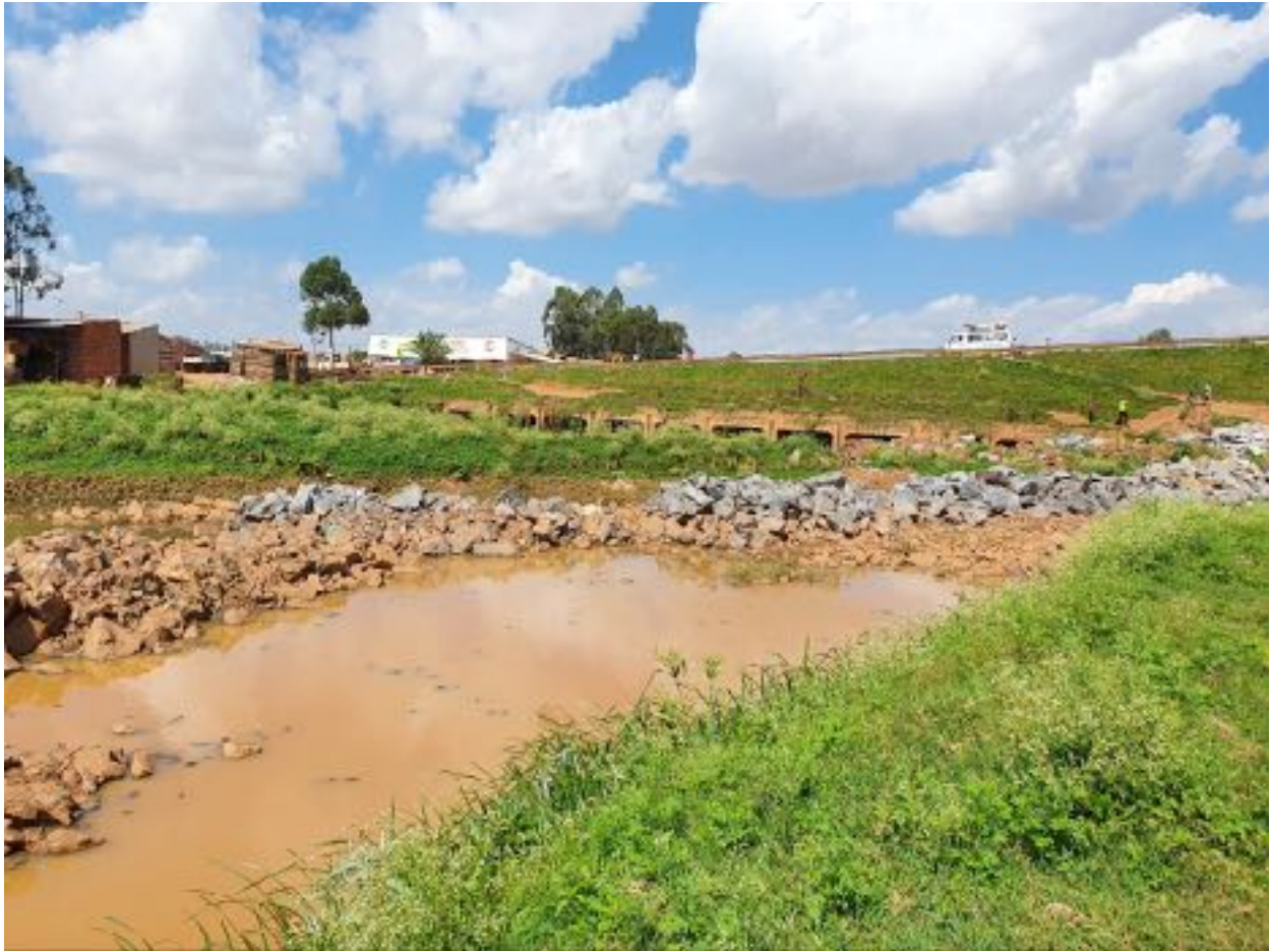
Figure 9 State of construction of the channel which is a risk for community members.
