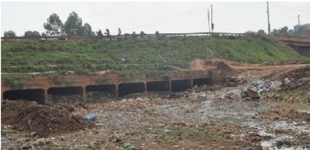
Picture 5: Silting of the box culverts at Kawaala Bridge (2021).
