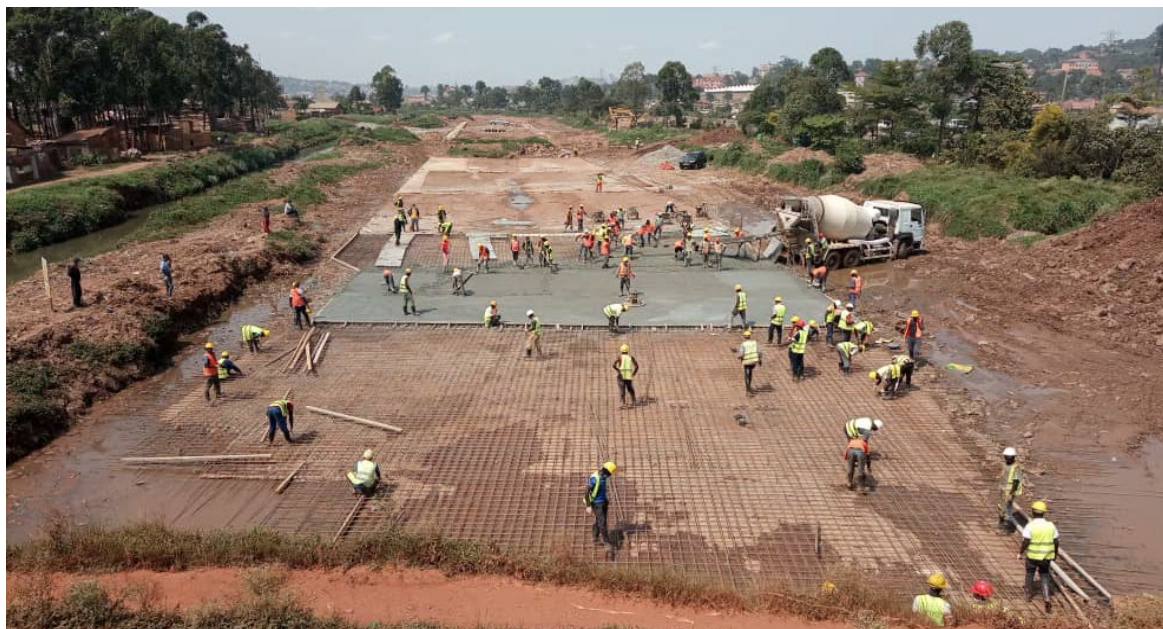
Picture 6: Silting of the Lubigi channel is being addressed through concrete lining of the channel in the Bwaise-Kawaala section where the works are ongoing (this is not the Kawaala-Hoima Section which pertains to the Request).
