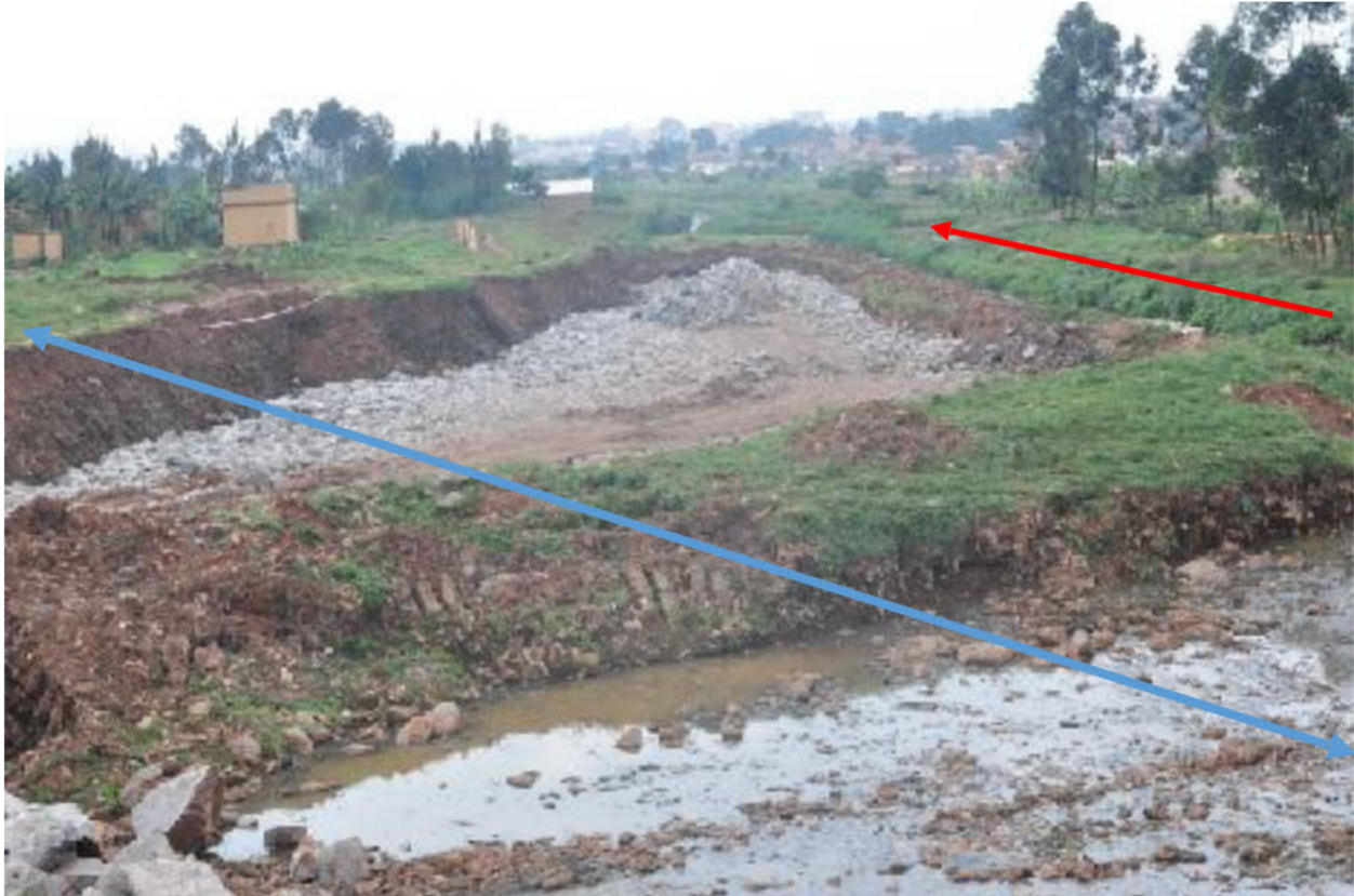
Figure 4 disturbed earth left from the construction of the channel diversion under KIIDP-1 (photo taken early 2021)
