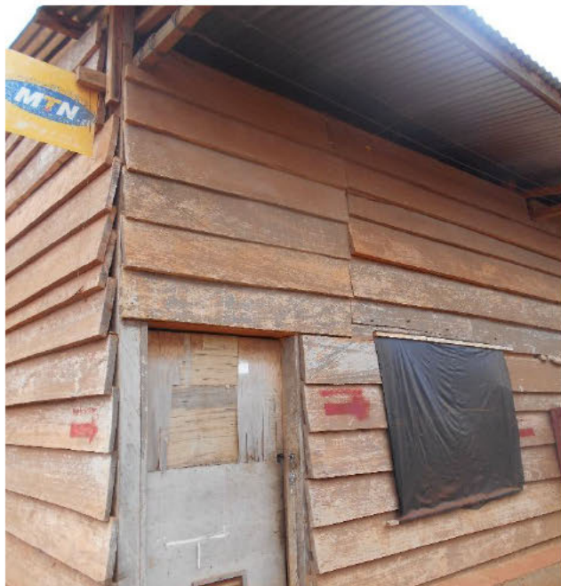
External view of employees’ house. Note that the window is blocked with black polythene paper to avoid dust and rains from pouring in.
