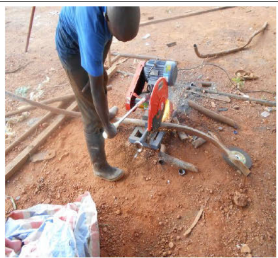
No welding goggles and gloves!
